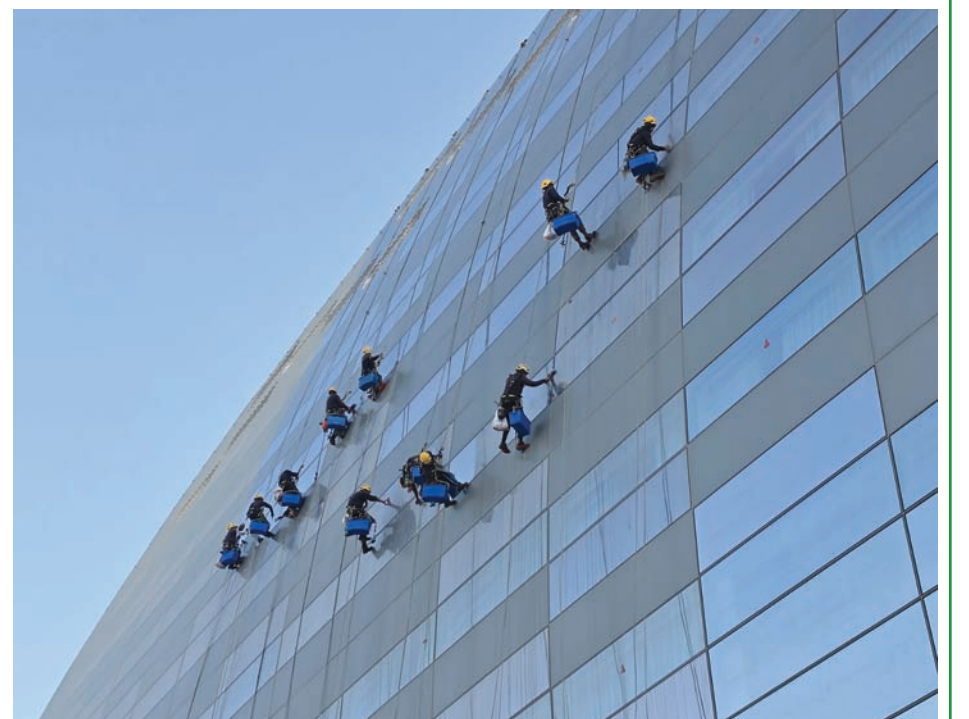
Suspended high above the ground, rope-access workers clean a building's facade in Doha.
