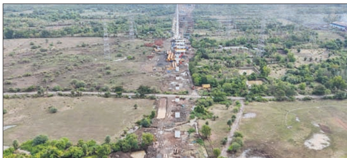
This aerial photograph shows the site of the Mumbai-Ahmedabad High Speed Rail project in Maharashtra's Boisar. (AFP)
