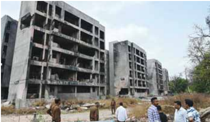
People stand near the damaged residential buildings at a site where Air India flight 171 crashed last year, in Ahmedabad yesterday. (AFP)
