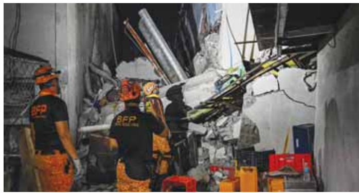
Responders assess a collapsed building after a 7.8 magnitude earthquake in General Santos City yesterday. (AFP)
