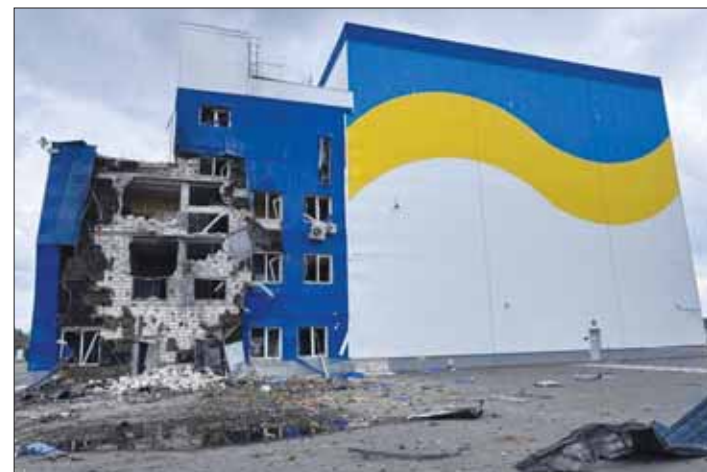
A handout image from Ukraine's Energoatom shows damage to a spent nuclear fuel storage facility, following what the company said was a drone strike, near Chernobyl, yesterday. (Reuters)
