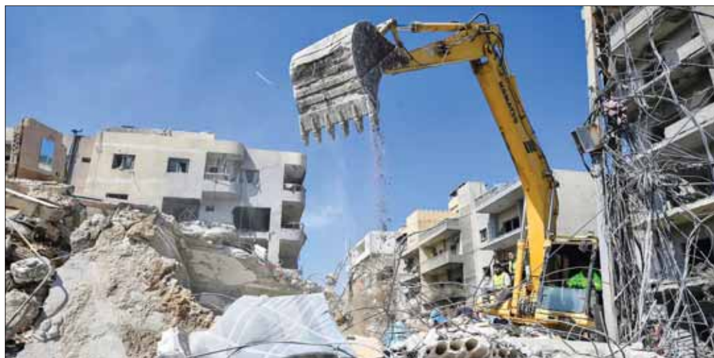
An excavator clears the rubble of a building as rescuers search for victims after an Israeli airstrike that struck near a hospital in Tyre. (AFP)
