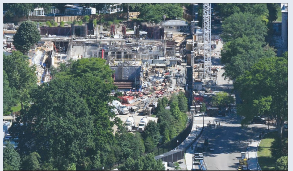
Construction is seen on the East Wing of the White House in Washington, DC, yesterday as part of US President Donald Trump's plans to build a White House ballroom. Trump showed off the site of his huge new White House ballroom on May 26, saying it would feature an underground military hospital and a "drone empire" on the roof. (AFP)
