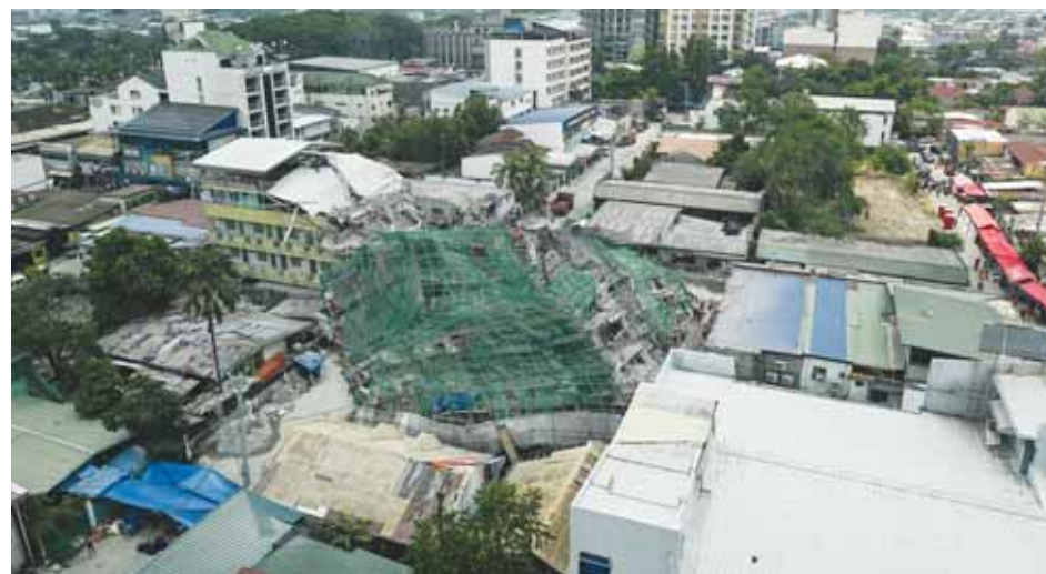
A view of the collapsed nine-storey building that was under construction in Balibago, Angeles City, Pampanga, yesterday. (Reuters)
