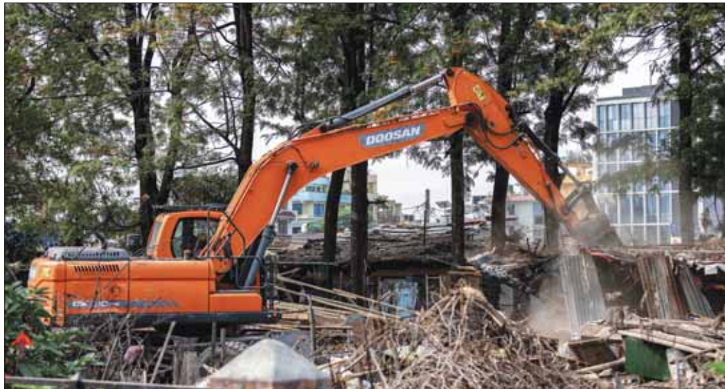
Nepali authorities demolish squatter settlements along the banks of the river Bagmati in Kathmandu yesterday. (AFP)
