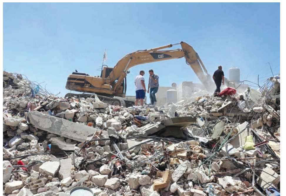
Resident Mohamad Ali Hijazi (left) stands next to an excavator clearing the rubble of destroyed buildings at a residential area in Tyre. - AFP
