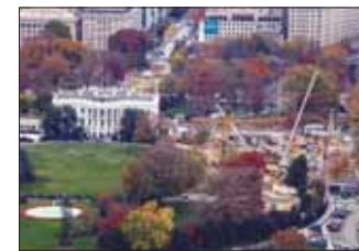
The demolition of the East Wing of the White House during construction of US President Donald Trump's proposed ballroom. (Reuters/File Photo)
