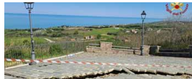
Damage caused by a landslide in a residential area in Petacciato, in the province of Campobasso. (Reuters)
