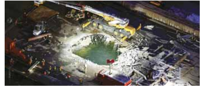
An aerial view of the site where three people were seriously injured and one is missing after falling about 40 metres from collapsed scaffolding at JFE Steel construction site in Kawasaki, south of Tokyo, yesterday. (Reuters)
