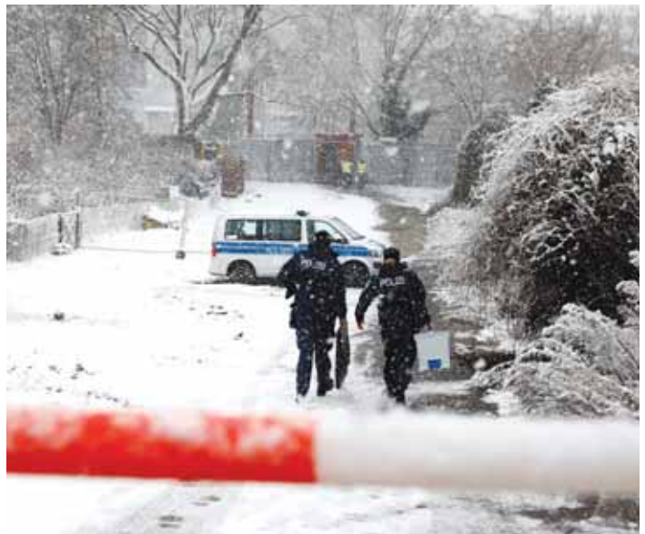
Police officers are seen outside a power distribution system that caught fire, causing a blackout in parts of the city, in Berlin. - Reuters
