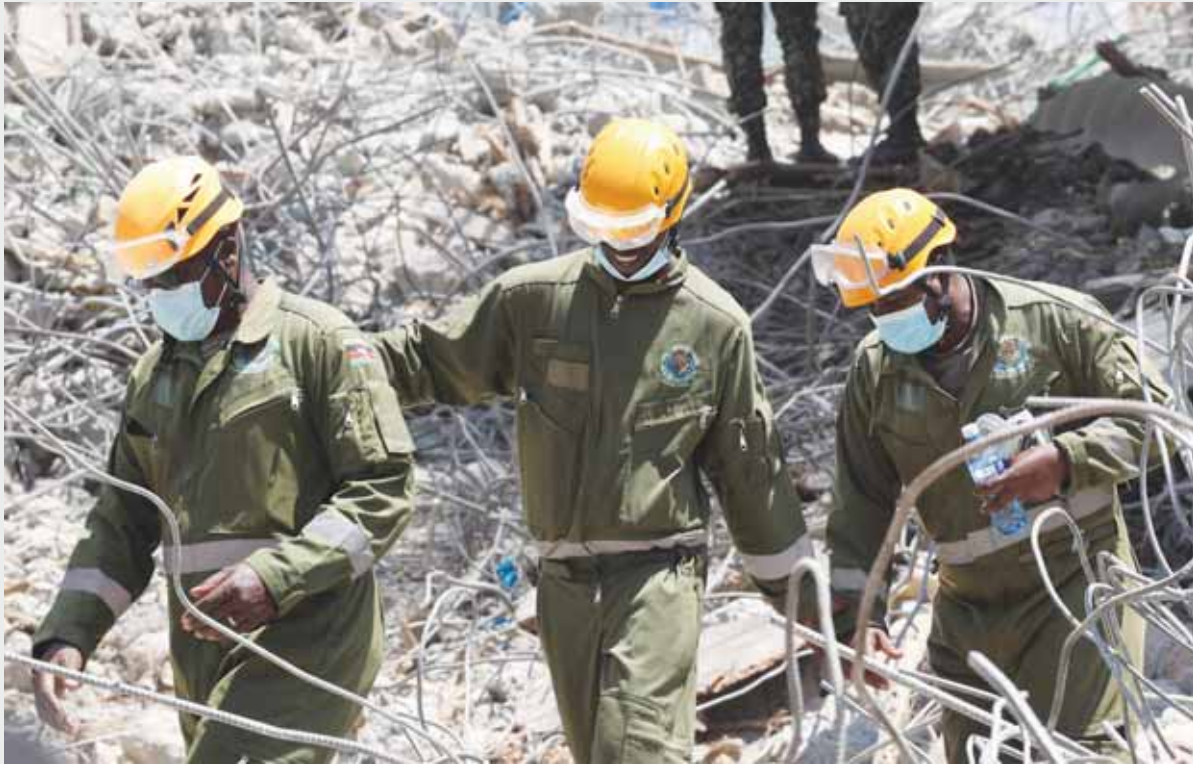
Rescue workers work at the site where a 16-storey residential building under construction collapsed near the shopping centre in the South C neighbourhood of Nairobi, Kenya yesterday.
