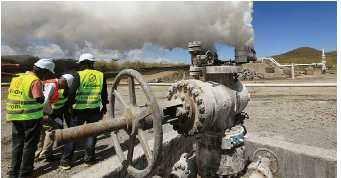
File photo: Kenya Electricity Generating Company (KenGen) workers are seen at a section of the Olkaria IV Geothermal power plant near the Rift Valley town of Naivasha.
