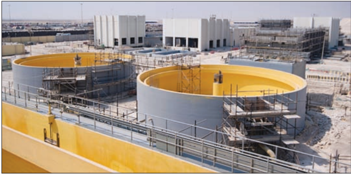
A view of the wastewater treatment facility.
