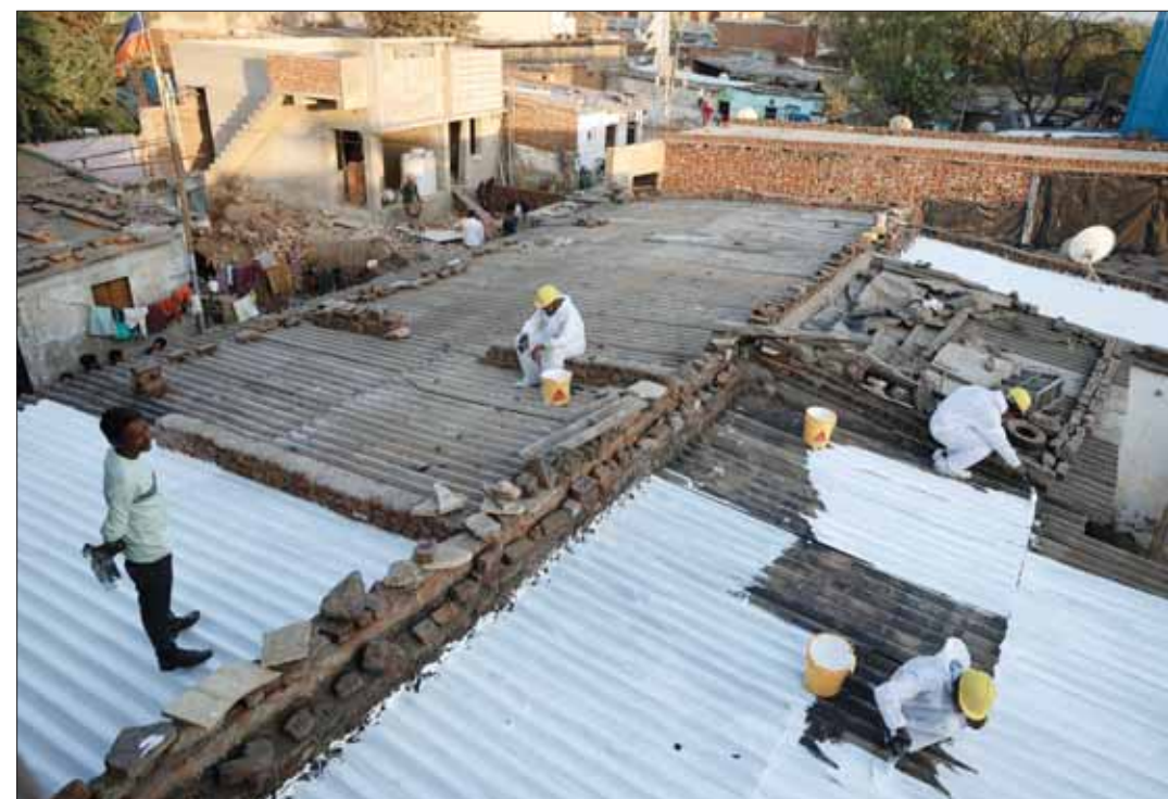
Painters apply liquid-applied membrane coating that according to the authorities helps to bring down the temperature inside the shanties at a slum in Ahmedabad. (Reuters)
