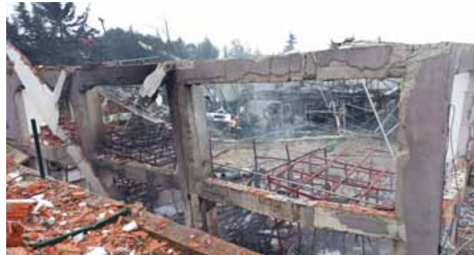
Firefighters work on the scene after a blast at an explosives factory in Balikesir, Turkiye. (Reuters)
