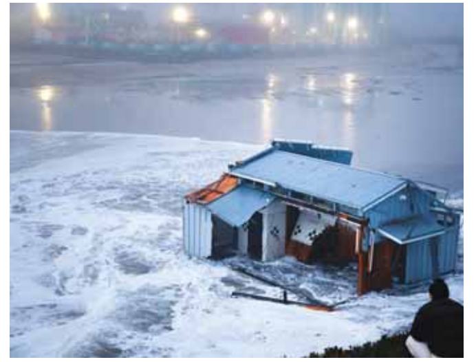
People look at the collapsed pier at the Santa Cruz Wharf in Santa Cruz, California. (AFP)
