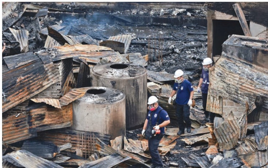
Police forensics personnel search for clues on the rooftop at the site of the deadly fire at a guesthouse in Porto Alegre.
