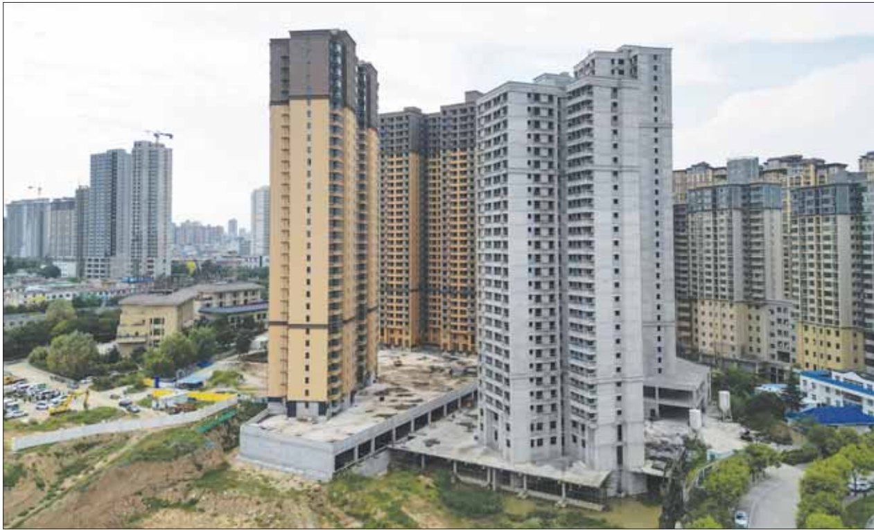
An aerial view shows unfinished residential buildings of the Gaotie Wellness City complex in Tongchuan, Shaanxi province. China's factory output and retail sales grew at a faster pace in August, but tumbling investment in the crisis-hit property sector threatens to undercut a flurry of support steps that are showing signs of stabilising parts of the wobbly economy.
