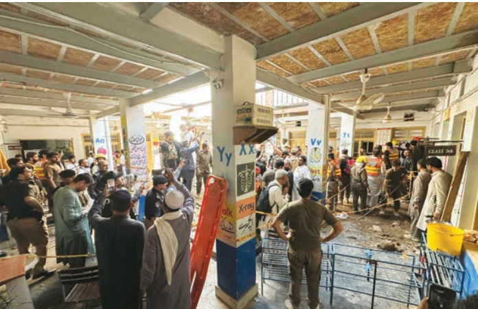
Rescue workers and residents gather after a school roof collapse in Peshawar, yesterday. (Reuters)
