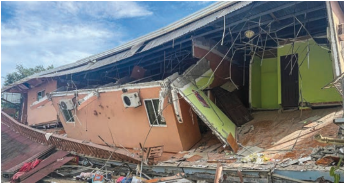
A collapsed house in Tonosi, located near Panama City. (AFP)
