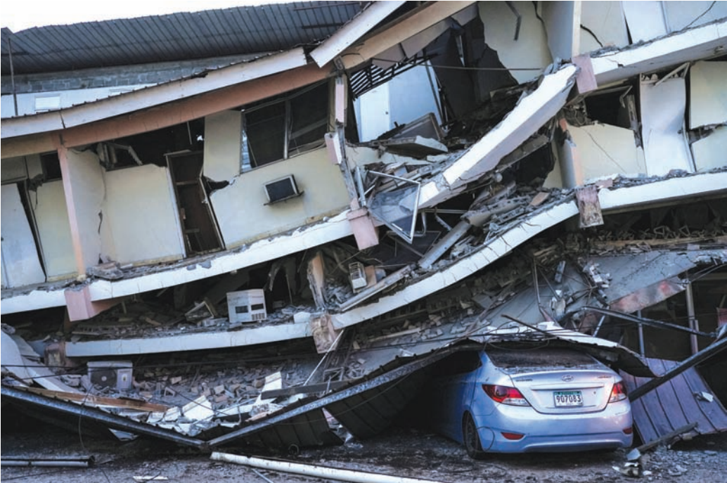
A car sits crushed beneath debris from a collapsed building after an earthquake struck near the southern coast of Panama, in Penonomé. (Reuters)
