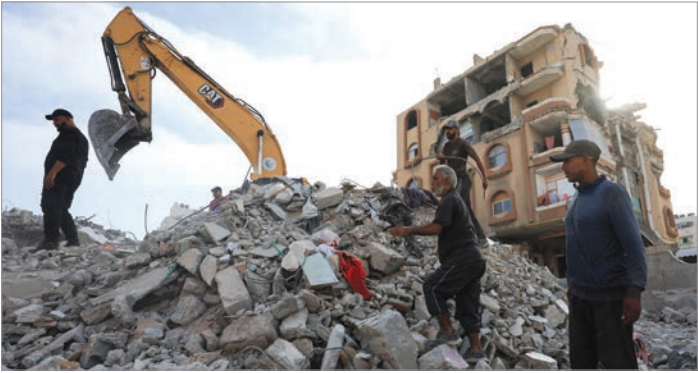
Palestinians inspect the rubble of a residential building that had been damaged in a previous Israeli strike during the war and collapsed on Wednesday, in Gaza City, yesterday. (Reuters)
