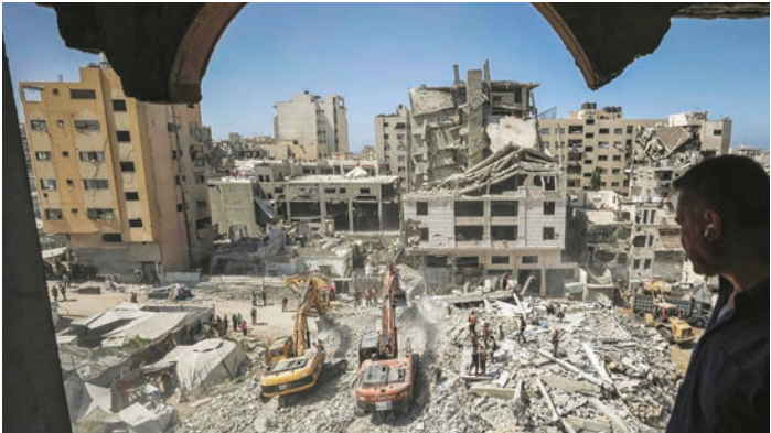
Rescuers excavate rubble to retrieve bodies from a collapsed building in the Tal al-Hawa area of Gaza City. (AFP)
