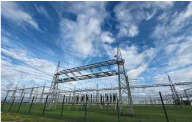
A power grid installation in Dormagen, in the western state of North Rhine-Westphalia, Germany. (Reuters)
