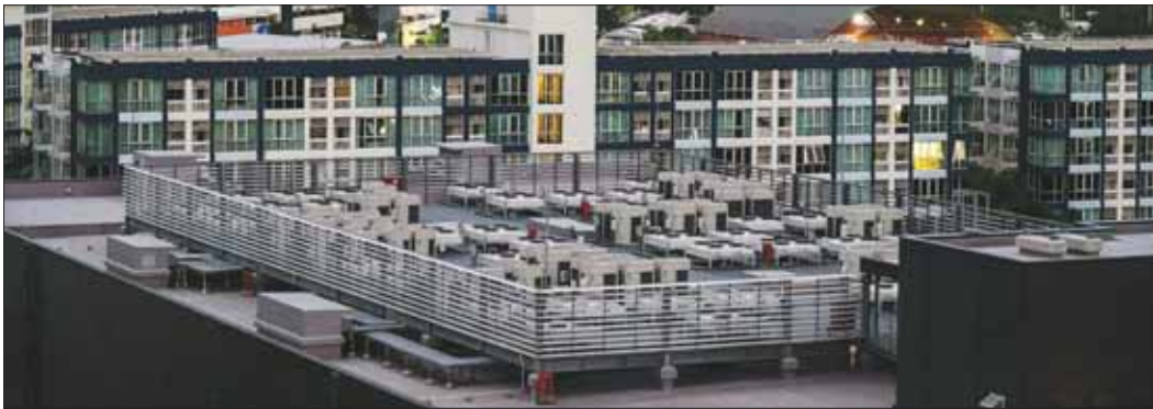
Cooling installations are seen on the rooftop of a data centre building in Bangkok yesterday. (AFP)
