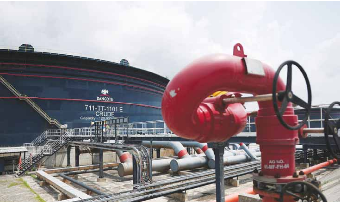
A crude oil tank is seen inside the Dangote Industries oil refinery and fertiliser plant site in the Ibeju Lekki district of Lagos, Nigeria. The listing will test investor appetite for one of Africa's most ambitious industrial projects.
