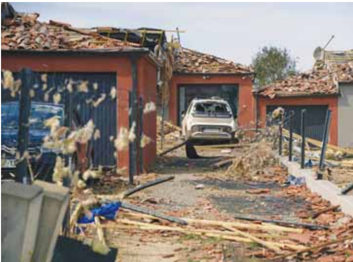
Damaged residential buildings following a tornado in Pomas, southwestern France. (AFP)
