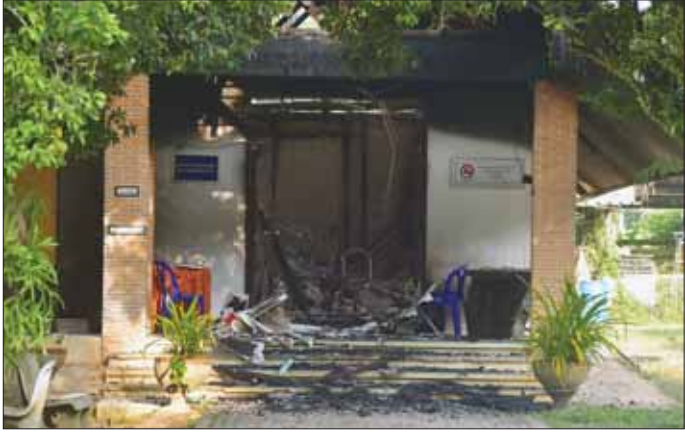
Fire damage is seen at a building in the Bongor Subdistrict Administrative Organisation office in Ra-ngae district in the southern Thai province of Narathiwat yesterday. (AFP)
