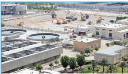
Sewage Treatment Projects
