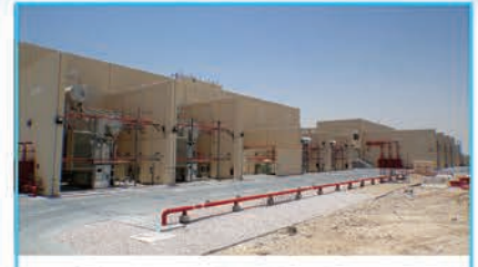
Kahramaa Substation Projects
